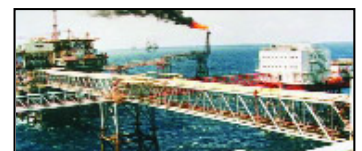
The project involved the design, fabrication and installation of process piping, commercial piping/plumbing and HVAC.
